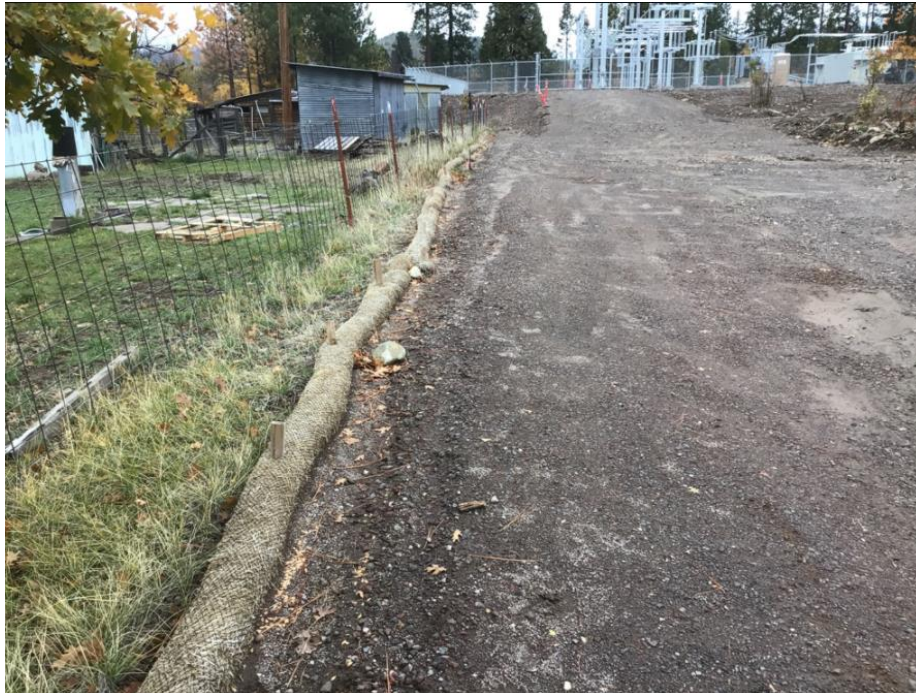
Photo 4: SWPPP erosion control BMPs (fiber rolls) were observed in good condition along the project boundary in accordance with APM WQ-1.
