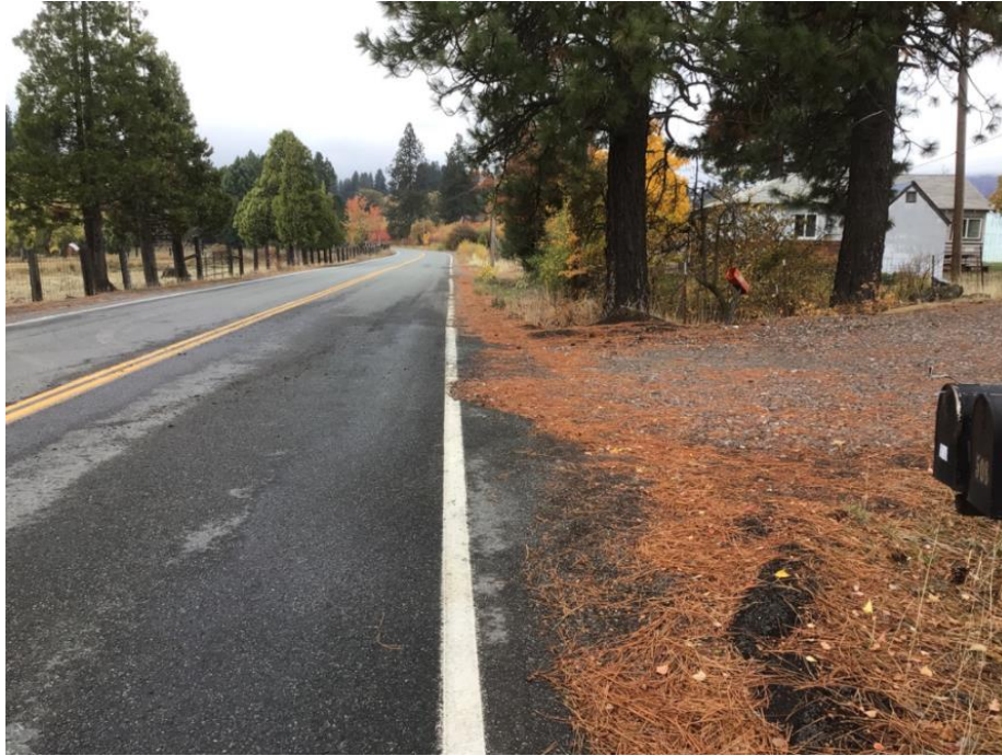
Photo 5: The stabilized construction entrance (gravel base) was observed in compliance with the SWPPP (APM WQ-1).
